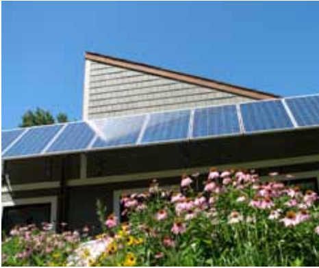
Solar panels at the Nature Center
